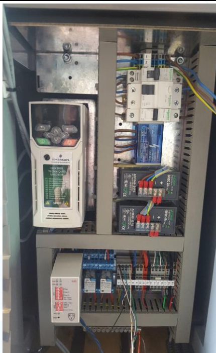
Picture 4 - Control cabin
