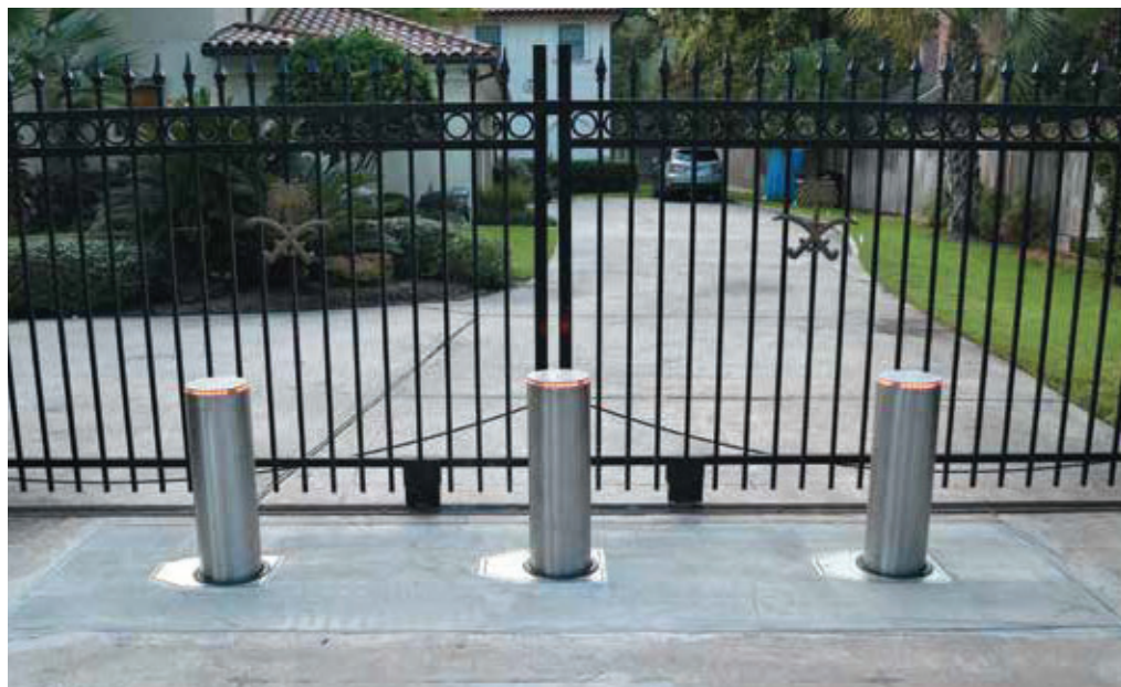
Retractable bollards, protecting an ornamental slide gate and the residence inside the gates. The bollards have LEDs along the top rim to increase their visibility.
